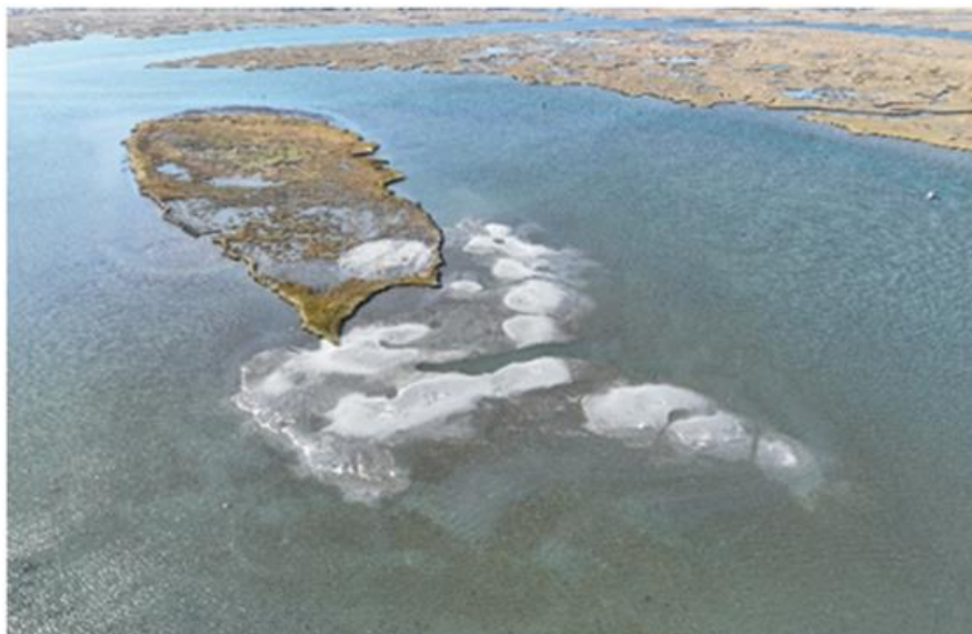
Fig. 5. Strategic placement of sandy materials to build marsh edge protection feature at Sturgeon Island.
