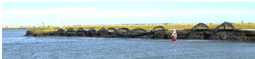
Fig. 3. Trialing techniques to build elevation and marsh edge protection with cohesive sediments at Sturgeon Island using a sediment distribution pipe.
